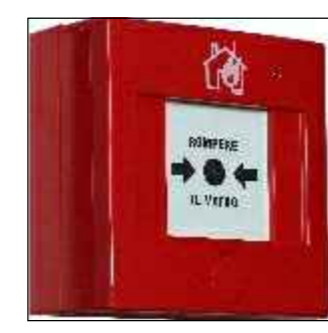
Manual call point for fire alarm recessed in the wall above 30cm the floor.
